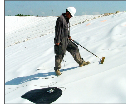
Leak Detection Liner
