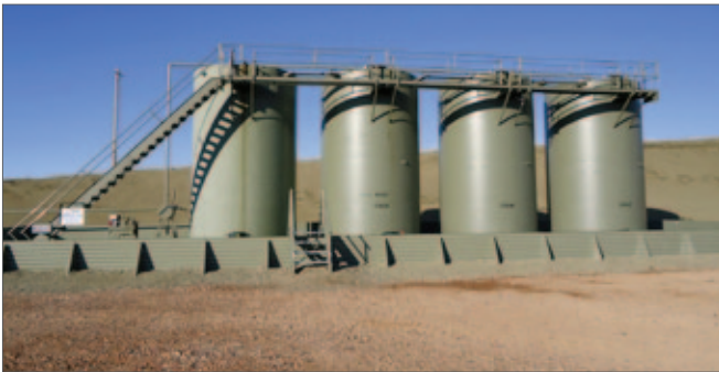
[Secondary Containment Tank Battery]
