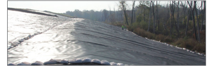
Used for Drainage
